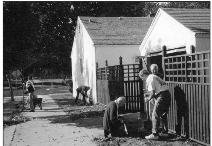
1997 Fence Construction (L to R): Arito Komure, Tom Kashiwagi, George Matsuoka, Steve Hill, Shiro Tokuno
